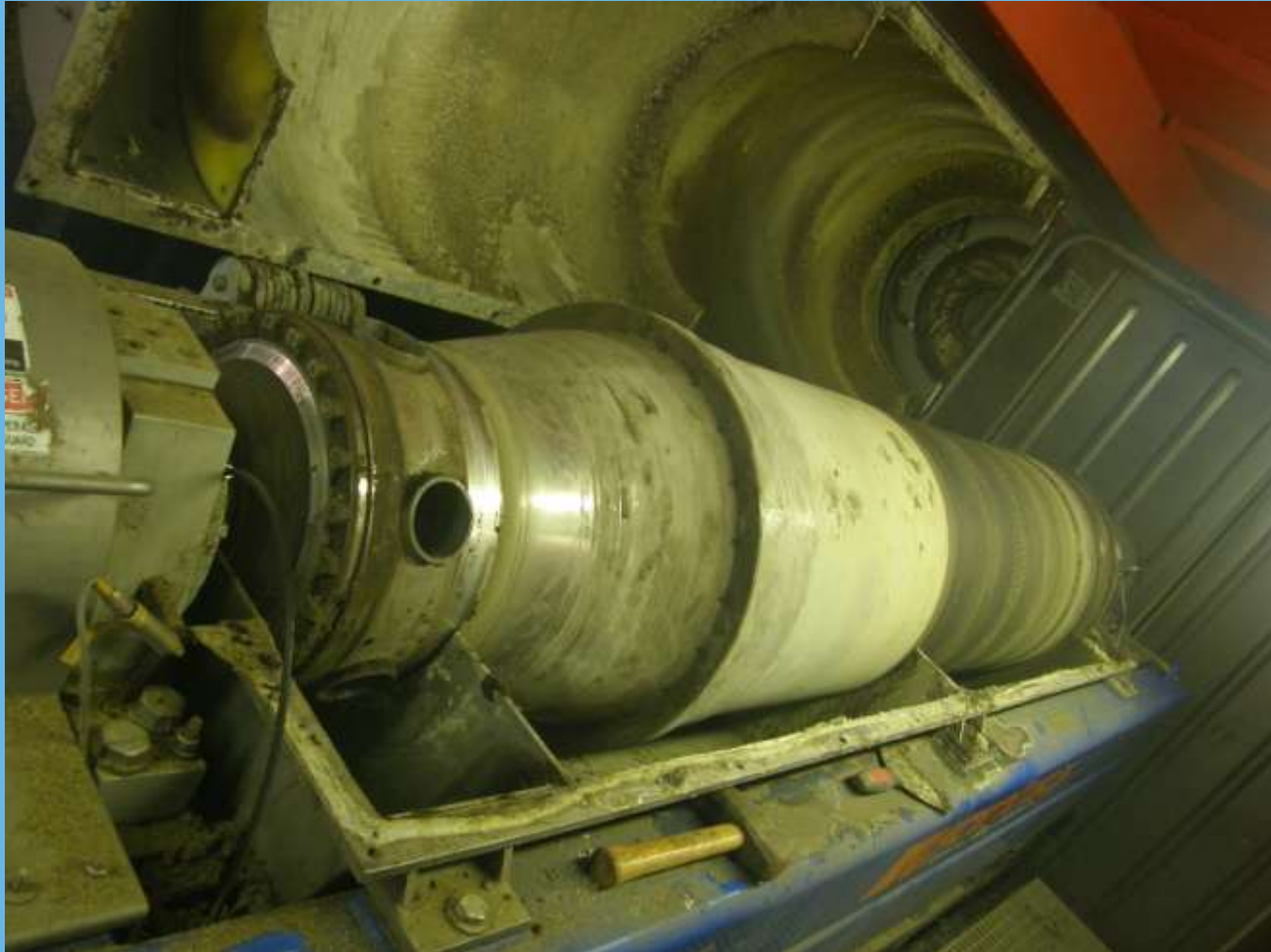
Centrifuge at the Dane County Digester; Clear Horizon
